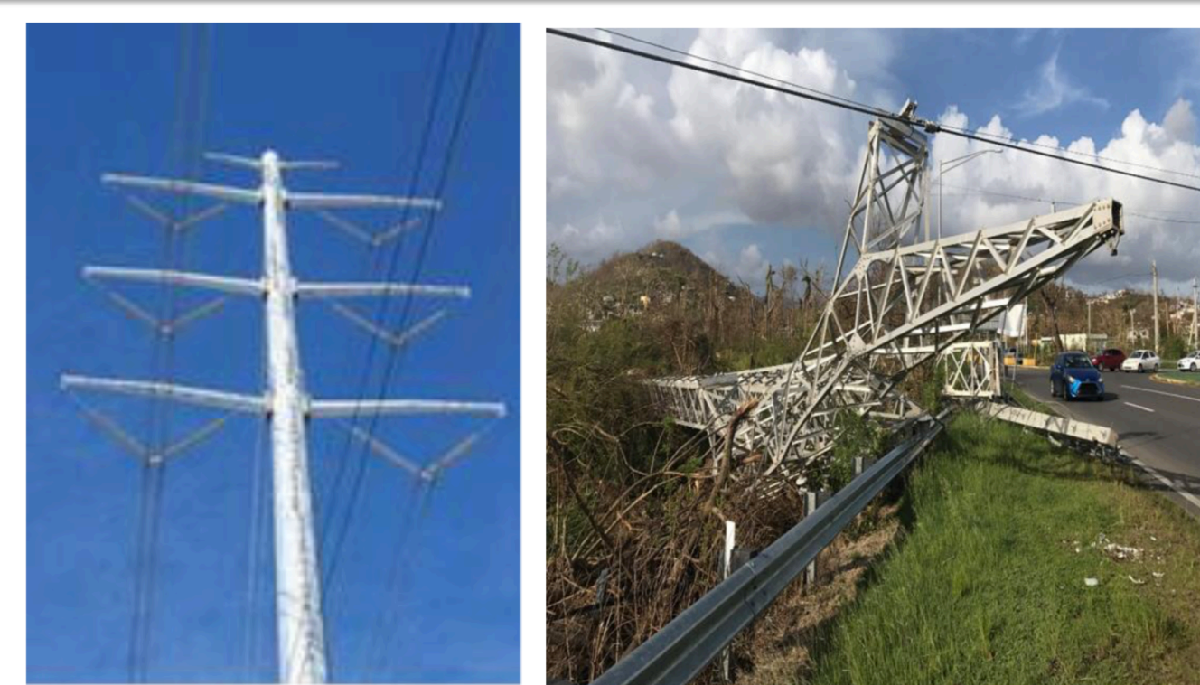
Monopole designs generally performed better than lattice tower designs. Source: NYPAC/Con Edison Damage Assessments
